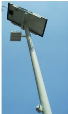
Figure 4: Solar LED Parking lot lights
