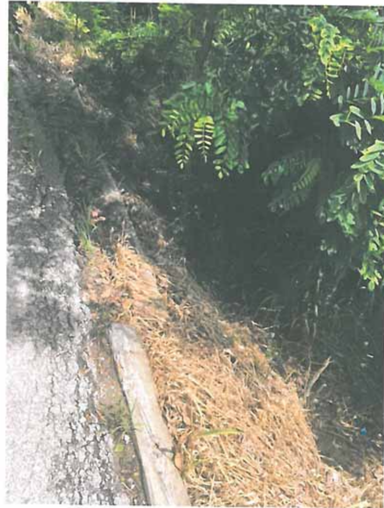
Edging/retaining wall giving way
