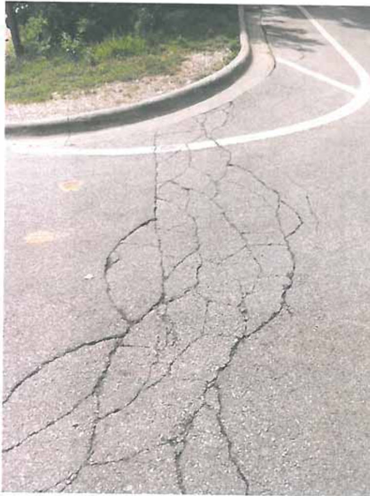
Movement in Roadway
